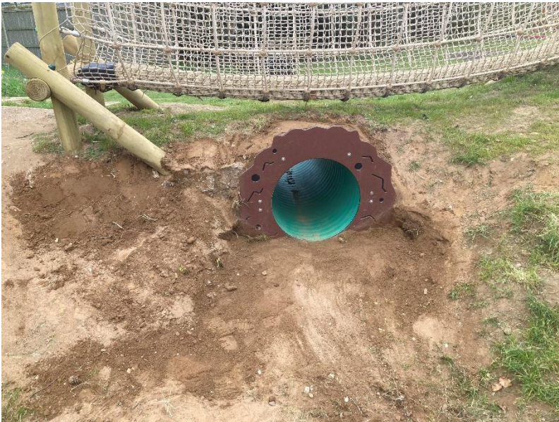
My initial attempt to re-instate the soil to stop any further possible water erosion
